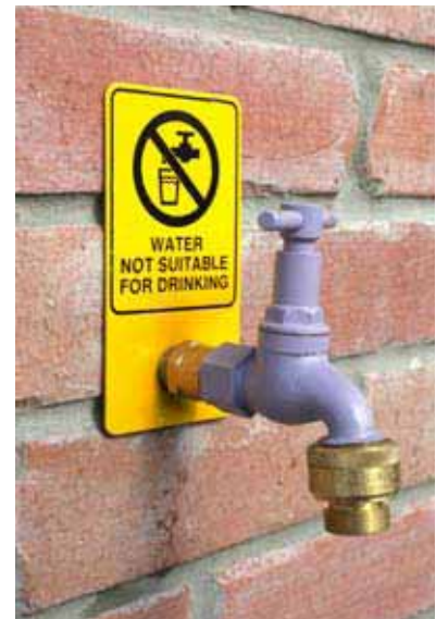
A purple Class A+ recycled water tap with a warning sign
