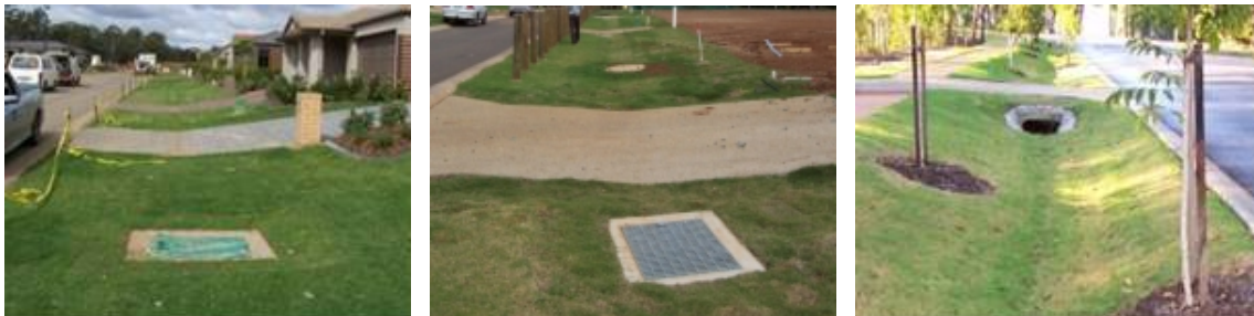
Plate 13.3-C: At-grade (left) under construction with trees yet to be established, pre-constructed 'at-grade' (centre) and elevated driveway crossings to allow vehicle access across swales
