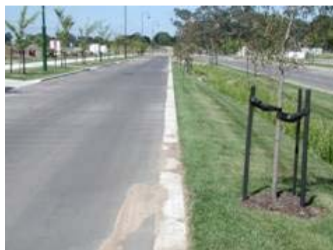
Plate 13.3-F: Flush kerb without setback, showing sediment accumulation on road
