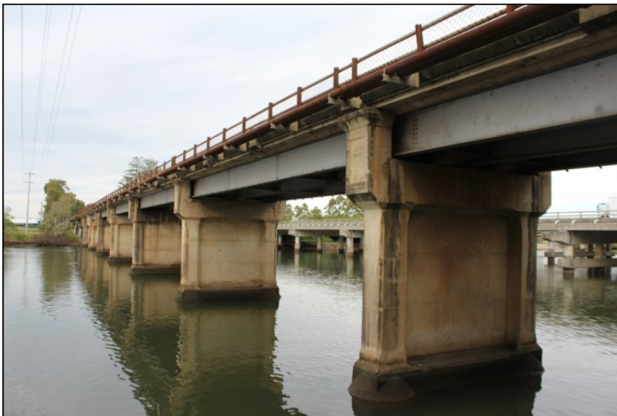
Coomera River Bridge 2016, view looking south. Image courtesy of City of Gold Coast.
