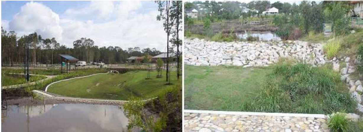
Plate 13.5-D: Spillway outlet weir structure of sedimentation basins at the Gold Coast and Coorparoo
