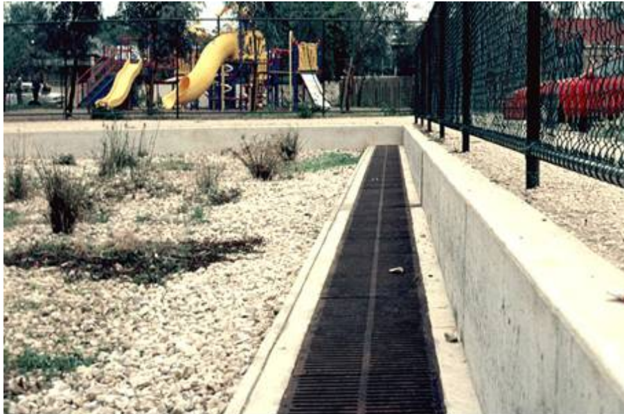
Infiltration System in Adelaide, showing the overflow trench
