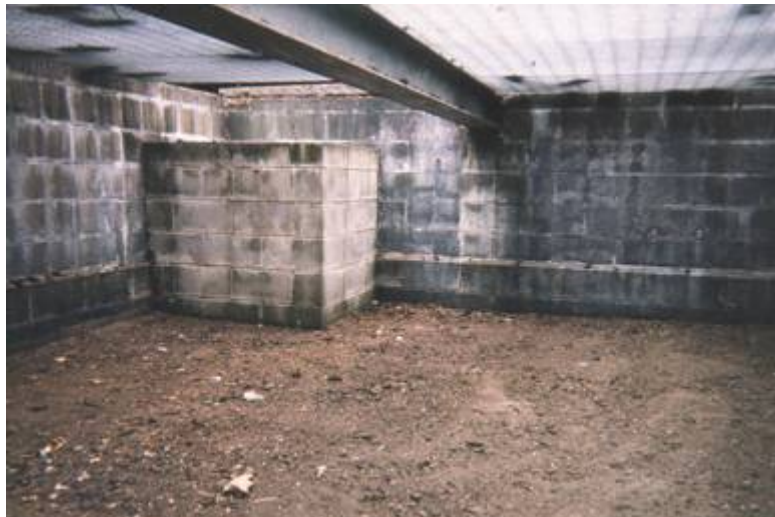
Figure 13.9-B: Underground Sand Filter (with overflow chamber in corner) for a Car Park in Auckland, New Zealand
